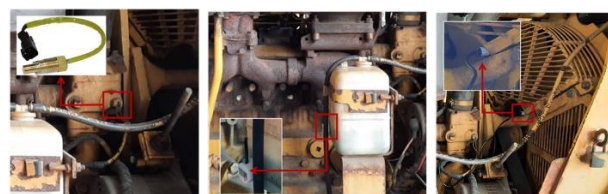
Fig. 10. Temperature, level, and speed sensor location.
