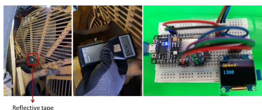
Fig. 7. Fan speed sensor working test.
