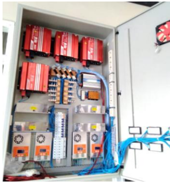
Figure 5: Electric panel box containing electric components of four groups of solar PV-Battery hybrid systems.
