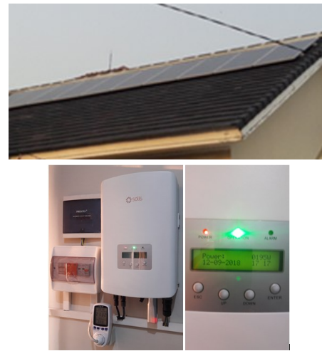
Fig 3. Installation of a rooftop solar panel PV system on site for the test.
