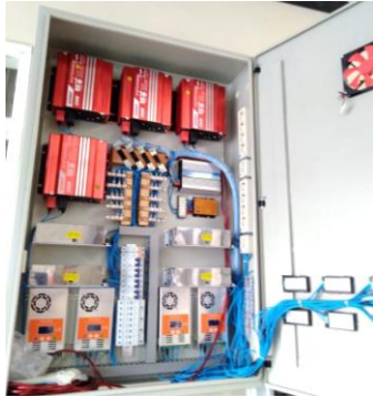
Figure 5: Electric panel box containing electric components of four groups of solar PV-Battery hybrid systems.
