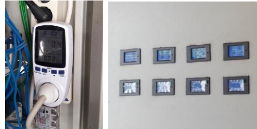
Figure 9: AC and DC power meters.
