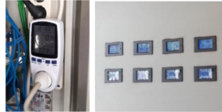
Figure 9: AC and DC power meters.
