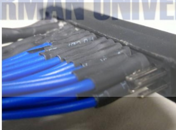
Figure 3-10 A6Con1 pin covered with heatshrink
